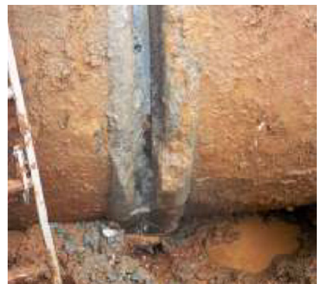
Leaking 6' PCCP main
