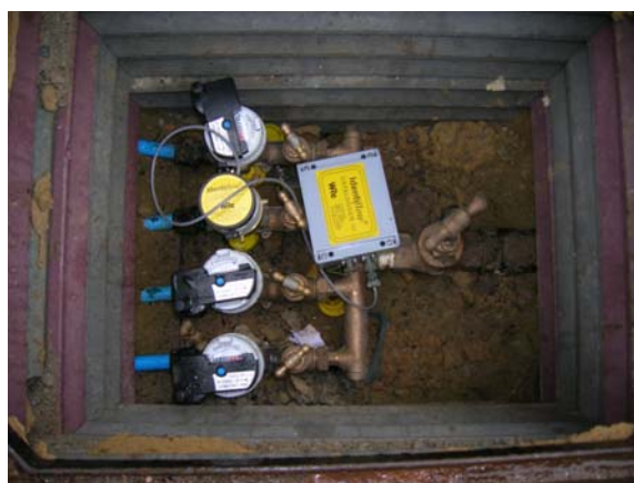
Identiflow ® in action – monitoring flow into a flat
